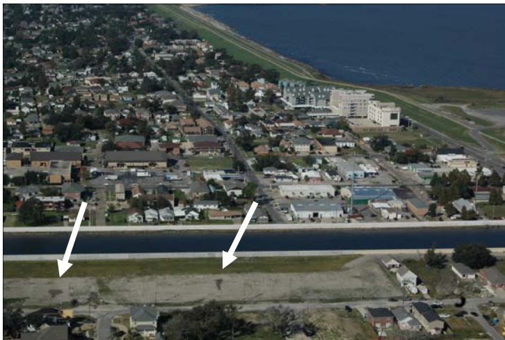
The arrows indicate the areas, near the 17th Street Canal levee, where two seepage spots were seen recently. The Corps is trying to determine the source of the water seepage. Simultaneously, the Corps is coordinating with its partners to bring on an independent peer review team to render an opinion on the affects of the seepage at this location. (USACE Photo)
