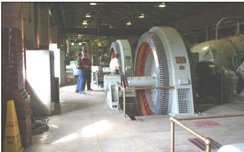
Members of the Corps' Project Delivery Team inspect re-wound motors at Orleans Pump Station #6. These motors were installed in 1915, were damaged by Hurricane Katrina, and repaired recently by the Corps of Engineers. They are again in superb working order. (USACE Photo)
