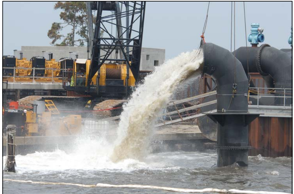
This photo, taken last summer, shows pumps being tested at the 17th Street Canal. New pumps on order for 17th Street and London Avenue Canals will dramatically increase pumping capacity at both outfall canals. (USACE Photo)
