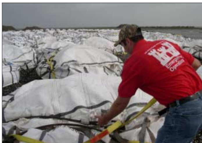
Jeff Richie, a New Orleans District project engineer, inspects cables used to attach 7,000 pound sandbags to helicopters for delivery to overtop sites. (Photo by Hank Heusinkveld, U.S. Army Corps of Engineers)
