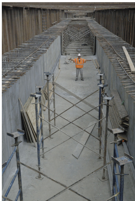
Left: Inspector Robert Martin stands in the 11ft x 14ft box culvert prior to placing the top slab at the Dwyer Pump Station Intake Canal construction project.
