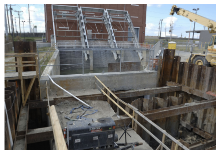
Above: Rainfall flows will be collected in the drainage canals and pumped from the Dwyer Pump Station into the Industrial Canal. The open evacuation and the required temporary retaining structure is shown in the foreground with the completed Dwyer Pump Station in the background.
