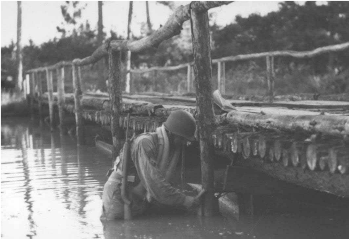
Figure 70. Placing dynamite to practice demolishing bridge at Fort Bragg, NC, undated (post-WWII) (NARA College Park, RG 111-SC WWII, Box 95, Photo SC147013).
