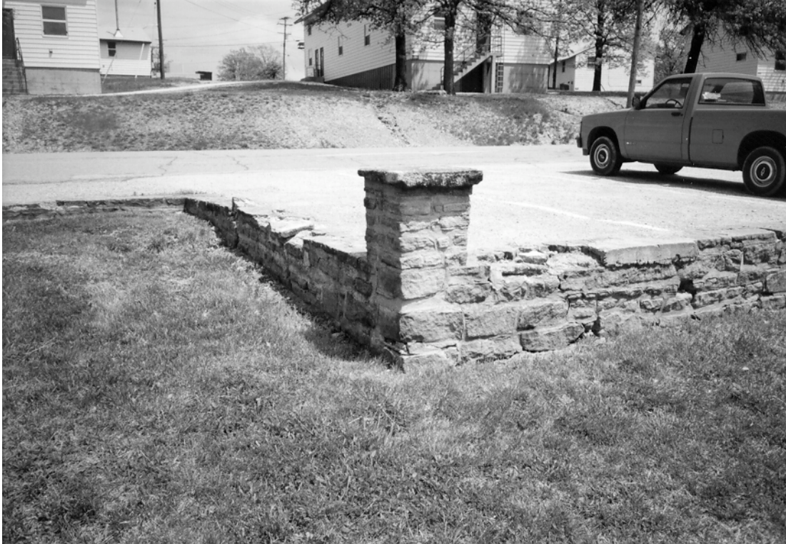
Figure A-4 Corner of Wall in Front of Building 2101 (courtesy, DPW Fort Leonard Wood).
