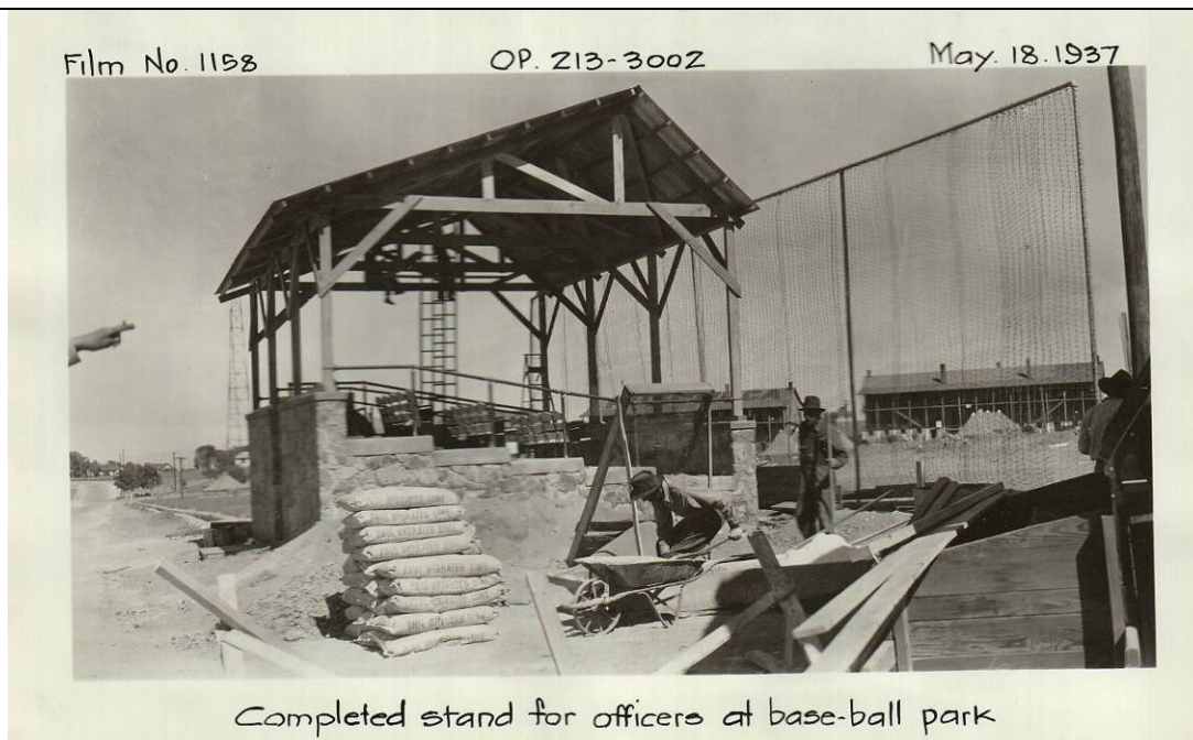
Figure 4-6. Officers' Grandstand under construction. From WPA Photo Album, Fort Huachuca Museum and Archives.
