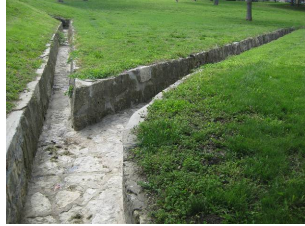
Figure 4-5: Y-junction of the rock-lined ditch. Terminus of the south arm of the ditch at upper left.
