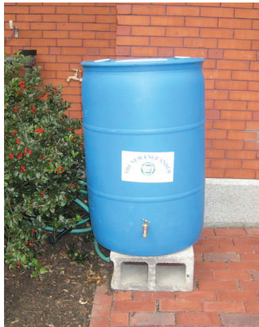
Figure 38: Cistern at Cambridge City Hall Annex
