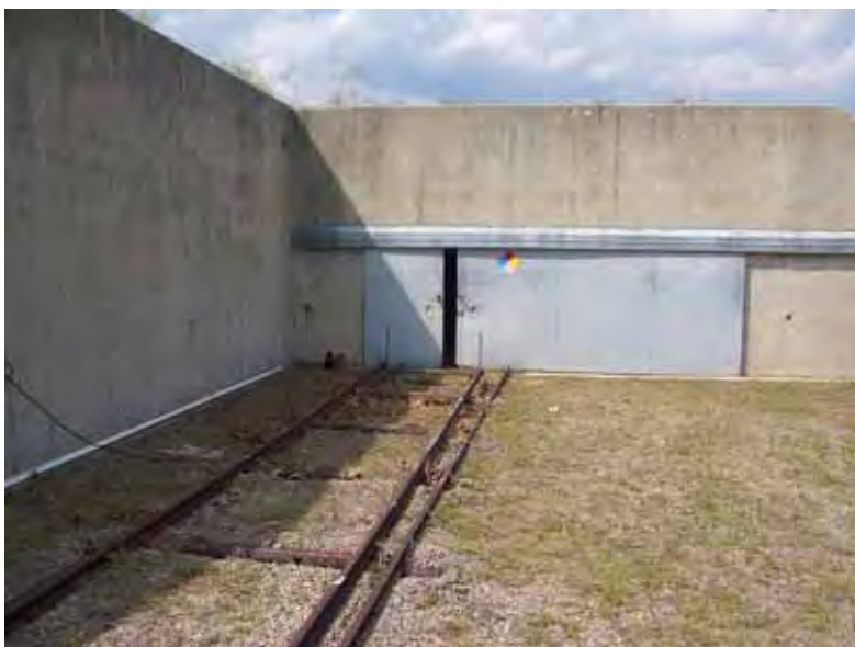
Figure 303. Target storage and repair building at the end of the target track built into an embankment, Fort Bragg, 17 May 2006.
