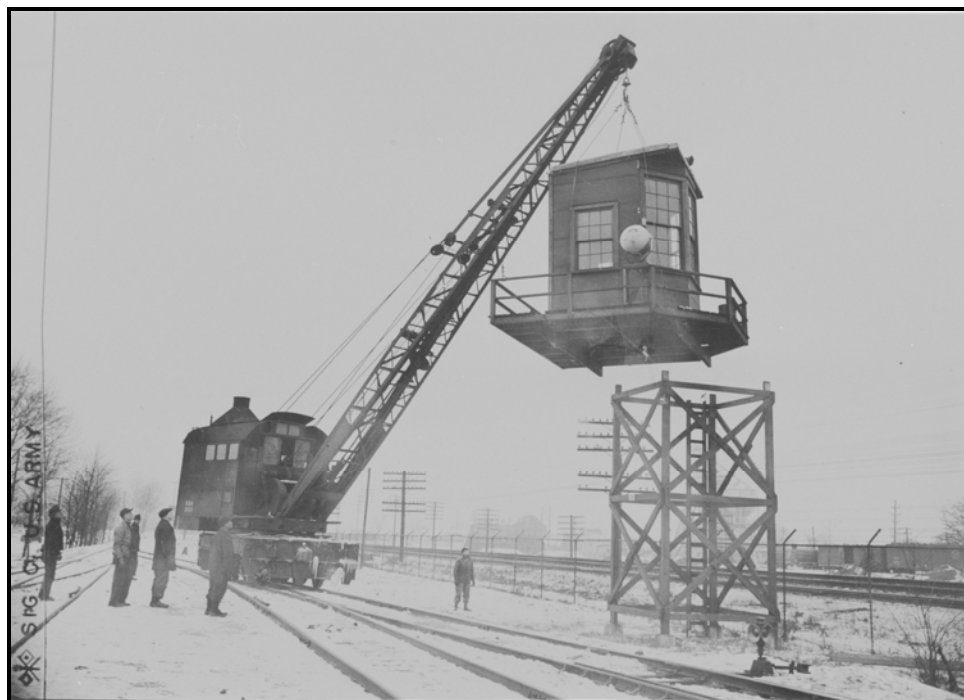
FIGURE 3-2. NEWER TOWER BEING MOUNTED AT THE COLUMBUS ASF DEPOT POW CAMP, FEBRUARY 1945 (NARA 1710-327850 [ROLL #2-33])
