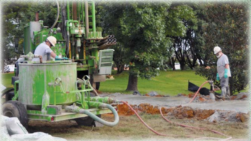
Contractors drill holes at Defense Supply Center Richmond, Va., for the installation of ground-source heat pumps. The new pumps are part of an energy-saving strategy to use about 50 percent less electricity than comparable air-source heat pumps.
