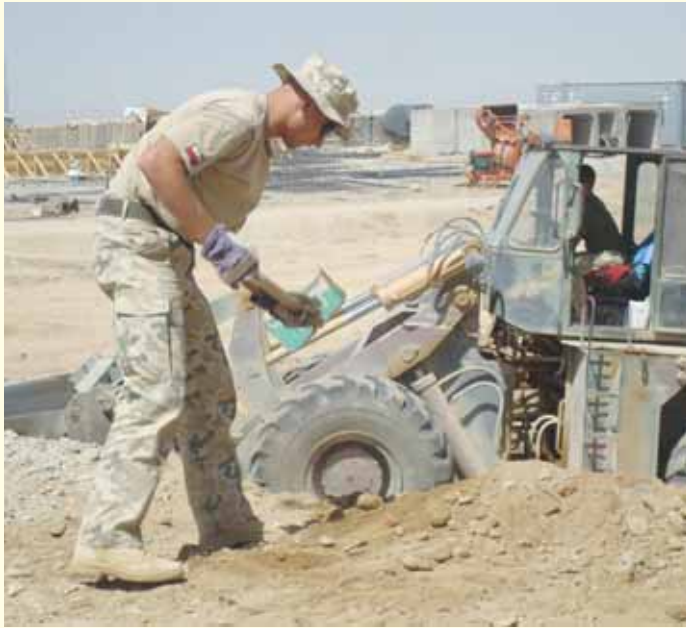
Polish Pvt. Piotr Oparski, Polish Engineer Platoon, works on the final touches of a culvert in Forward Operating Base Sharana, Afghanistan, as a scoop loader hauls the rest of the dirt
