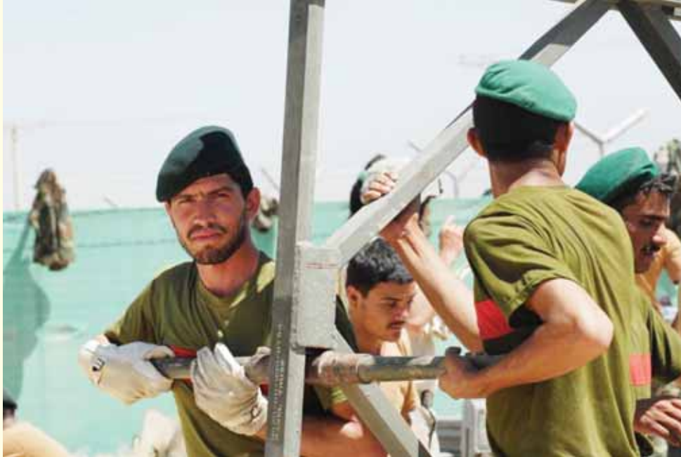
Afghan National Army Engineers of 4-3 Kandak, 201 st Corps Command, assemble a 40-foot Bailey Bridge in preparation for emplacement of a Bailey Bridge during future missions in Afghanistan.
