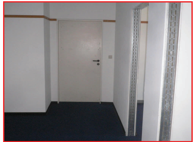
New offices for two Trial Defense Counsel (right) after the drywall construction was plastered and painted, and new “JAG blue” carpet was installed. The door above leads into the new Senior Defense Counsel’s office.
