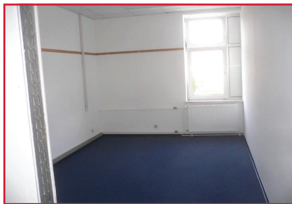
Existing three-panel windows had to be converted to one-panel, with the center panel replaced to accommodate the dividing wall. Radiators that ran the length of the windows were also replaced with smaller individual ones.
