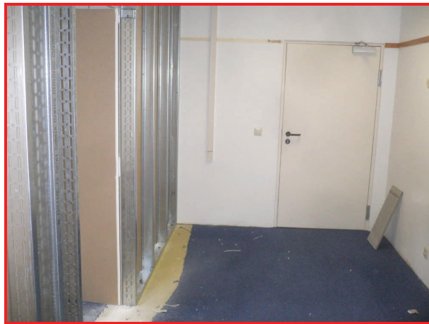
New Claims Examiner offices (left) under construction, in the room adjacent to our Claims Judge Advocate’s office. Contractors installed soundproof double-thick drywall and tore up and replaced the 10-year old carpet.
