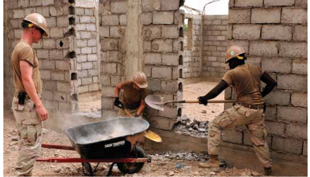
DJIBOUTI SCHOOL - Service members with Naval Mobile Construction Battalion (NMCB) 7 remove debris from Ecole 5, a five-classroom school in Djibouti on June 30, 2010. NMCB-7 is operating out of Camp Lemonnier, Djibouti. (U.S. Navy photo by Chief Petty Officer 2nd Class Nathan Laird)
