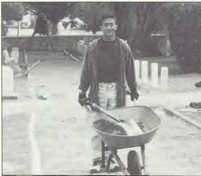
Army Sgt. Jose Ferrera, Headquarters Company, uses a wheelbarrel to move topsoil used to level the grave sites. (Photo by Capt. Susan Meyer)
