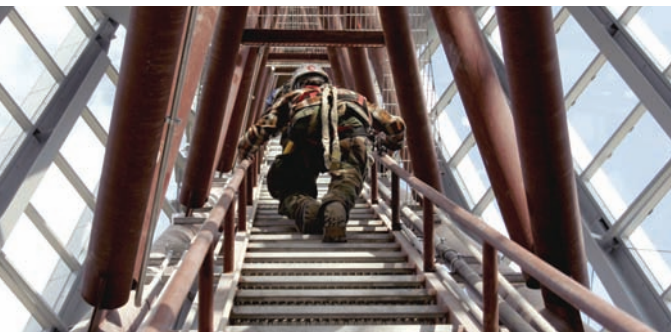
A construction worker climbs up the ladder in the center of the National Museum of the Marine Corps' mast to finalize some structural work at the 210 foot pinnacle of the museum at Quantico, VA.
