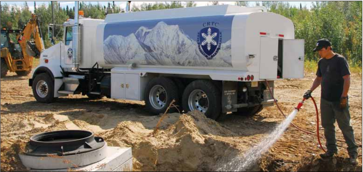
Heavy Equipment Operator Russell Hollembaek prepares a trench for an electrical conduit to one of the CRTC meteorology team's three new Sonic Detection and Ranging stations. Any type of construction is difficult or impossible to complete in winter, when the ground freezes to depths exceeding 10 feet.
