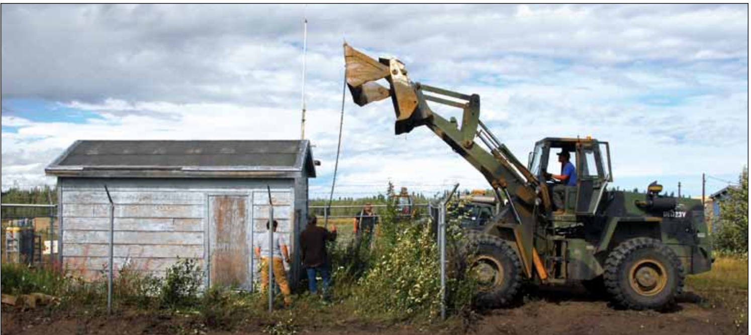
CRTC employees use heavy machinery to lift a meteorology building onto steel support beams. Alaska's extreme freezes and subsequent thaws often cause structures like this to sink into the ground. "Because of our remoteness, and because of many competing demands from the many other U.S. Army Alaska tenant units, it is not always possible to get the necessary, timely support from the department of public works to work on these types of projects," said CRTC Commander LTC John Cavedo.
