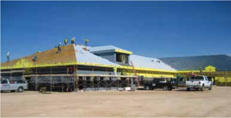
Roofing work progresses on the new child development center at Fort Bliss, TX, Dec. 9, 2010. USACE has expanded construction at the installation for the past five years as units of the 1st Armored Division relocate there from Germany. (Photo courtesy of USACE.)
