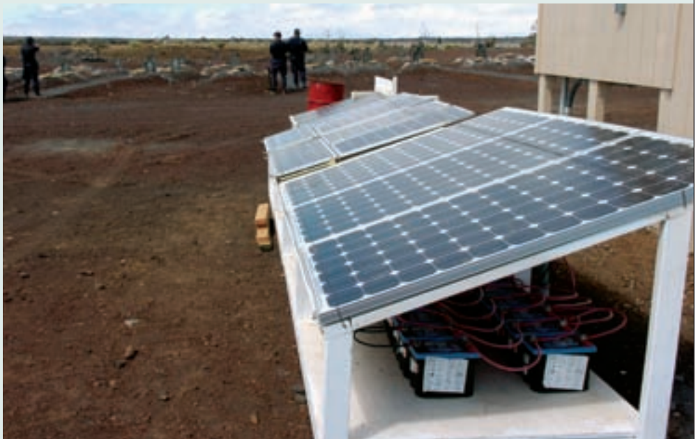
An example of Army energy efficiency is the solar panels at the Pohakuloa Training Area, HI, (shown here) that charge the batteries beneath them, which provide enough energy to operate the range tower building beside it and the range pop-up targets. (U.S. Army photo by Chicpaul Becerra, U.S. Army Garrison-Pohakuloa Training Area Public Affairs.)
