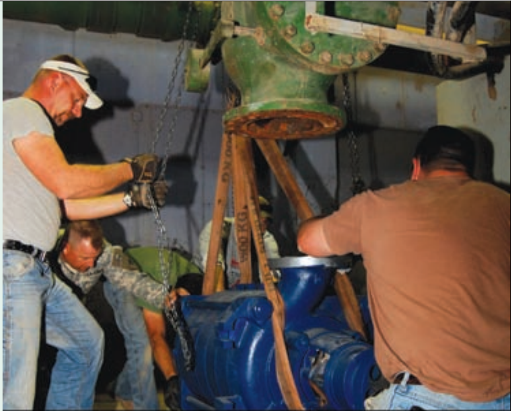
SFC Robert Roach, water operations NCO, 76th Brigade Special Troops Battalion, and contractors from Kellogg, Brown, and Root (KBR), wench a new, high-capacity, multistage centrifugal water pump into place at the Al Qayyarah pump house at the Tigris River Nov. 5, 2008, as part of a massive, joint project overseen by the 16th Sustainment Brigade (SB) to build water infrastructure in the drought-prone Ninawa region in northern Iraq. (U.S. Army photo by SGT Keith Anderson, 16th SB.)
