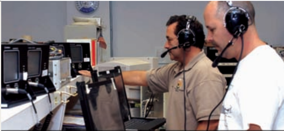
Technicians test a digital switching unit at a tactical operations center (TOC) at TAD. The testing is part of CECOM LCMC’s global field service representative support for 4ID, 1st Cavalry Division, Stryker brigades as well as the TOC reset mission for 4ID. (U.S. Army photo.)
