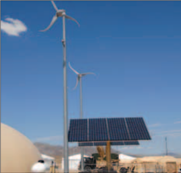
The Net Zero Plus Joint Capabilities Technology Demonstration on May 27, 2008, at the National Training Center, Fort Irwin, CA, showcased PM MEP's vast technologies across DOD, from small generators to solar power. (U.S. Army photo by Richard Mattox, PEO C3T.)
