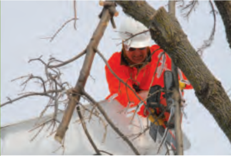
Because of swift and timely actions by the Fort Riley DOC to leverage the contracting resources, independent contractors from across Kansas converged on Fort Riley to assist with power restoration efforts after an ice storm caused power outages to 8,000 post residents in December 2007. Here, Joe Gerber, with A.A. Gifford Electric, Manhattan, KS, chainsaws broken limbs on Fort Riley, Dec. 15. ( Fort Riley Post photo by Dena O'Dell.)
