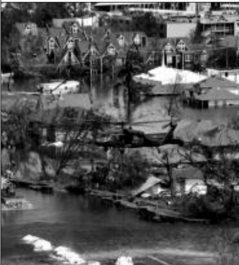
A Texas ARNG UH-60 Black Hawk helicopter drops a single 6,000 pound bag of gravel and fine material into the gap in the 17th Street Canal Flood Wall, New Orleans, LA. Texas ARNG helicopters cycled throughout several days to transport giant sandbags to help fill breached levee walls around the flooded city. (USACE photo by Alan J. Dooley, Hurricane Katrina Corps of Engineer Operations.)
