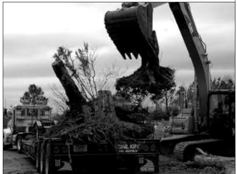
A contractor removes tree trunks uprooted during Hurricane Katrina as part of a massive effort by USACE to remove nearly 120 million cubic yards of debris — twice the amount collected during the Florida hurricanes in 2004. (U.S. Army photo by Daren Reehl.)
