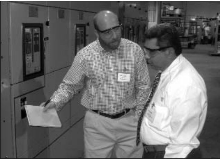
U.S. Army NETCOM/9th ASC Engineer Randy White (left) and Army Product Manager Defense Wide Transmission Systems (PM DWTS) Product Leader Jorge Blanco witness the successful acceptance testing of new power generation equipment for Okinawa, Japan, at the Caterpillar ISO plant in Alpharetta, GA, on Dec. 15, 2004. (Photo by Tim Kennedy.)
