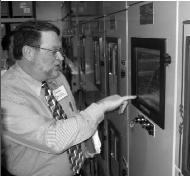
Jim Leander, Chief of the Okinawa DPW, tests the power generation equipment’s touch screen monitors, which give the operator the ability to “drill down” and virtually view any component. (Photo by Tim Kennedy.)
