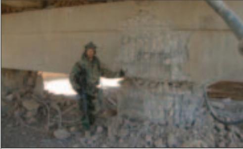
A Soldier with the 54th Engineer Battalion examines structural damage to a bridge spanning the Euphrates River. USACE engineers stateside provided a TeleEngineering bridge assessment to determine what repairs needed to be made to the support columns and how much load the damaged bridge could safely bear. (U.S. Army photo courtesy of USACE/GRD.)
