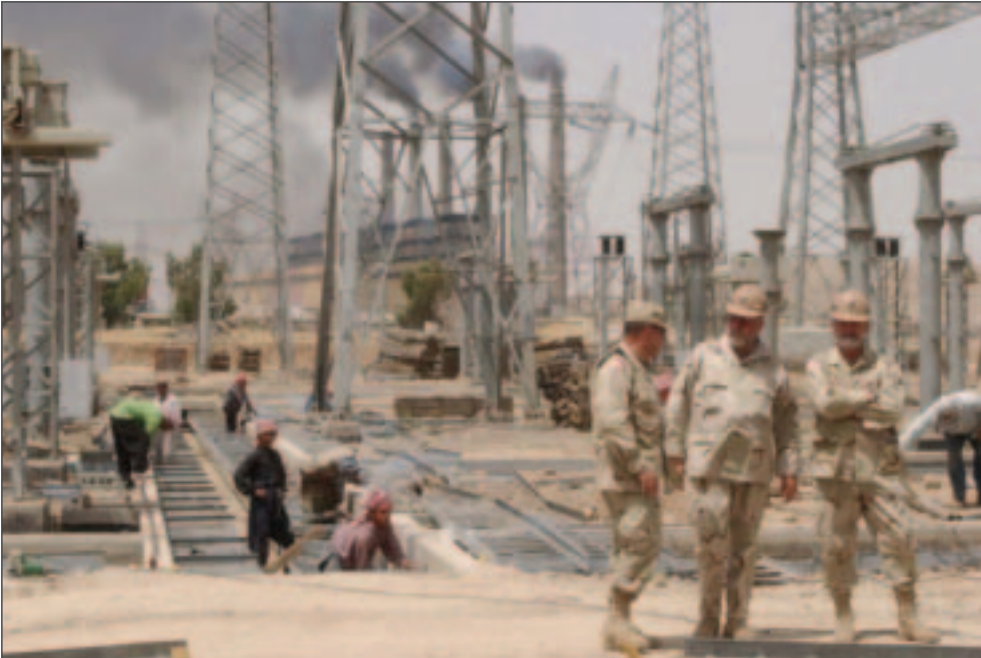
USACE personnel work with local Iraqi workers to construct new switching facilities to augment rehabilitated power generators to assist the coalition partnership in reaching its 6,000 MW power generation goal by June 2005. (GRD photo by Thomas A. O'Hara.)
