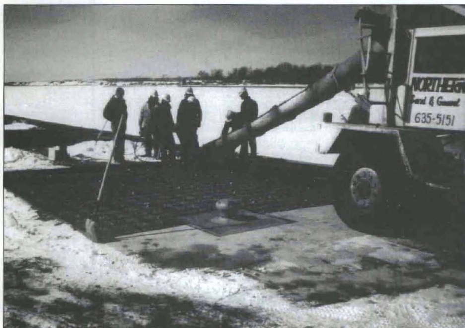
Demonstration of antifreeze admixture for concrete at Corps of Engineers Soo Locks in Saulte Sainte Marie, MI, during March 1994 with temperatures as low as -20 degrees C.
