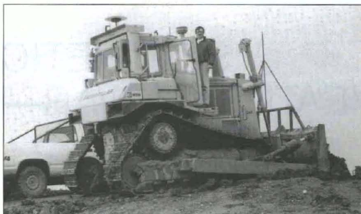
TEC scientist on a Caterpillar dozer uses GPS positioning information to automate construction activities.
