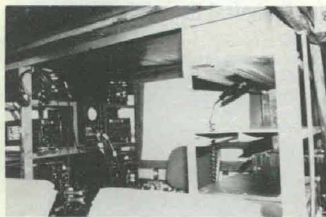
265th CEW Company members reduced AN-TRQ 32 weight by almost 10,000 pounds. Remodeled AN-TRQ 101 interior was designed with angle iron and metal shelving.
