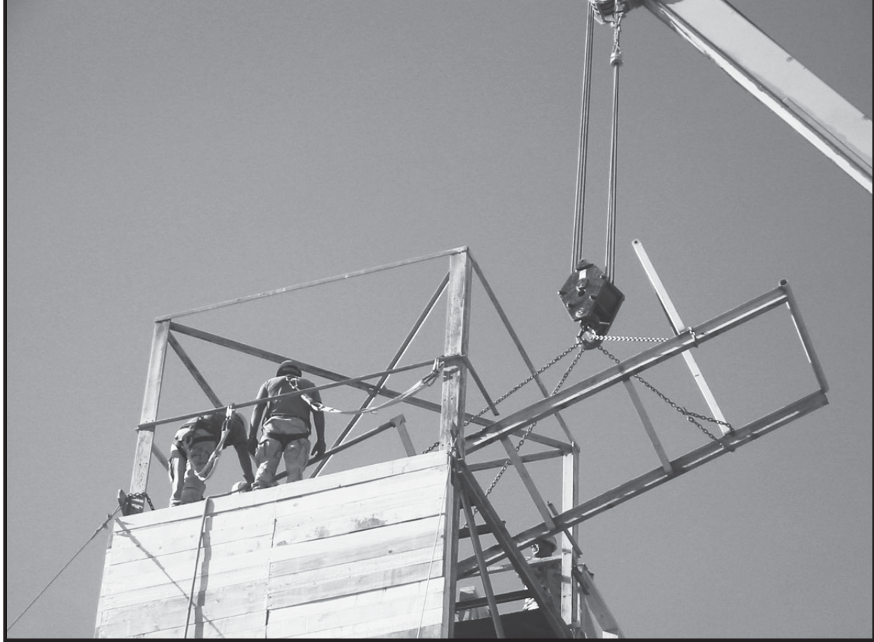
Charlie Company's maintenance personnel place the top platform of the main rappel tower.
