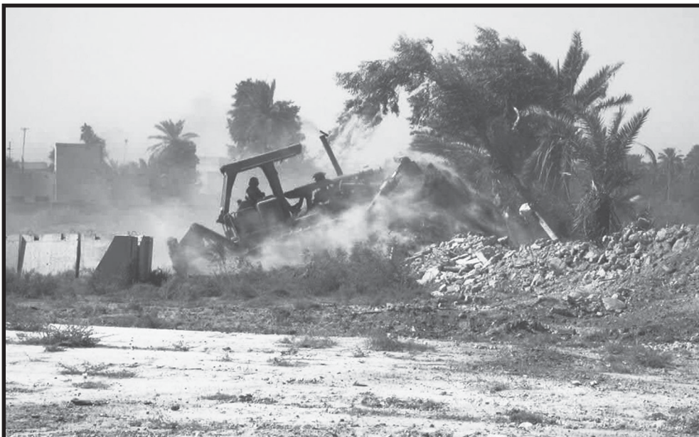
Engineers use a bulldozer to push debris into a protective berm around the logistical base.
