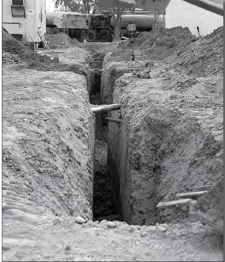
Unmarked buried utilities create a challenge for trenching operations during base improvements.
