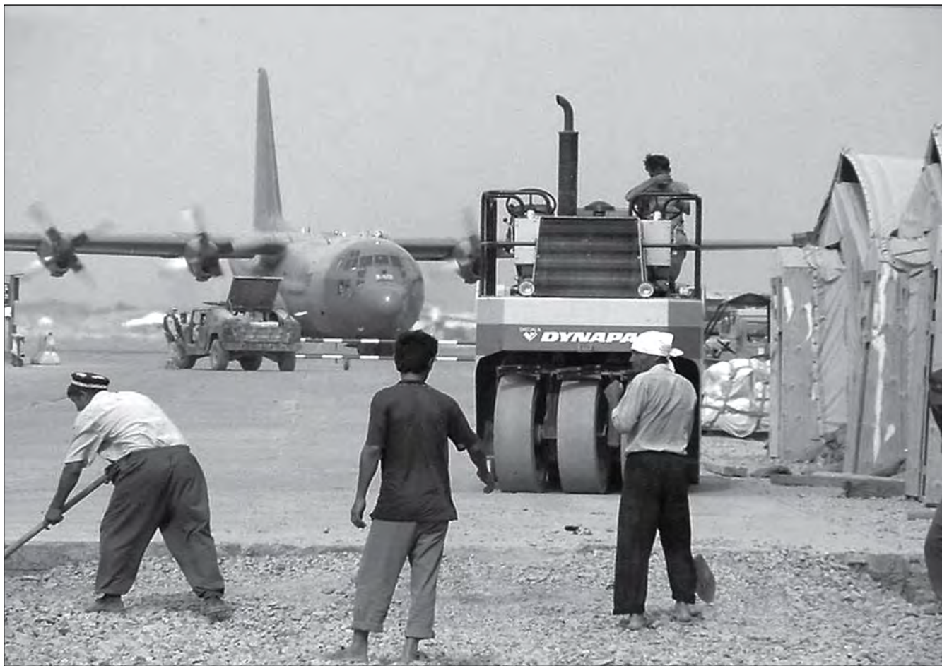
Road repair at K2 was a top priority in 2002 to improve theater logistics and airbase operations.
