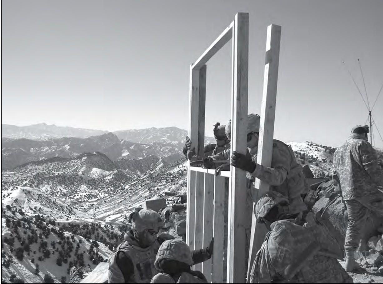
Engineers from Bravo Company, 864th Engineer Battalion, Fort Lewis, Washington, put up wall structures for a new bunker that will serve as an outpost in the middle of the mountains in eastern Afghanistan.
