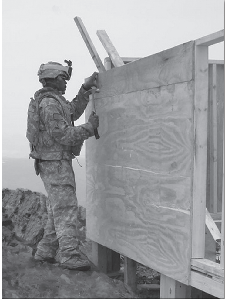
A Soldier from Bravo Company, 864th Engineer Battalion, Fort Lewis, Washington, nails the wall for a bunker at an outpost on an Afghanistan mountain.
