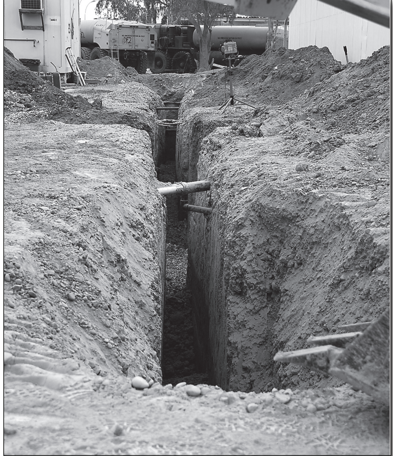
Unmarked buried utilities create a challenge for trenching operations during base improvements.
