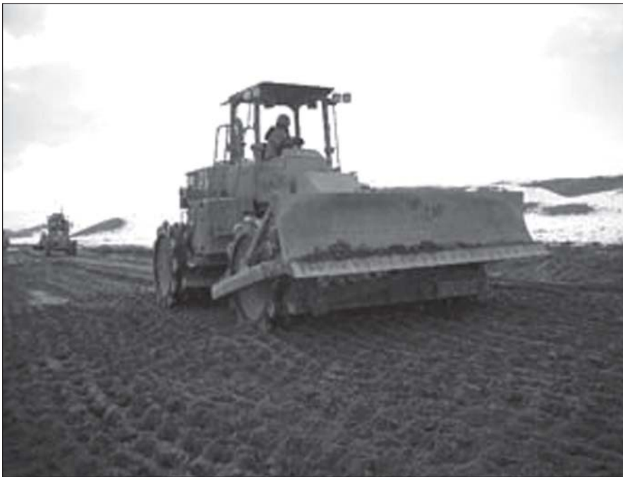
A high-speed compactor breaks up frozen chunks of soil and compacts it to strengthen the subbase.
