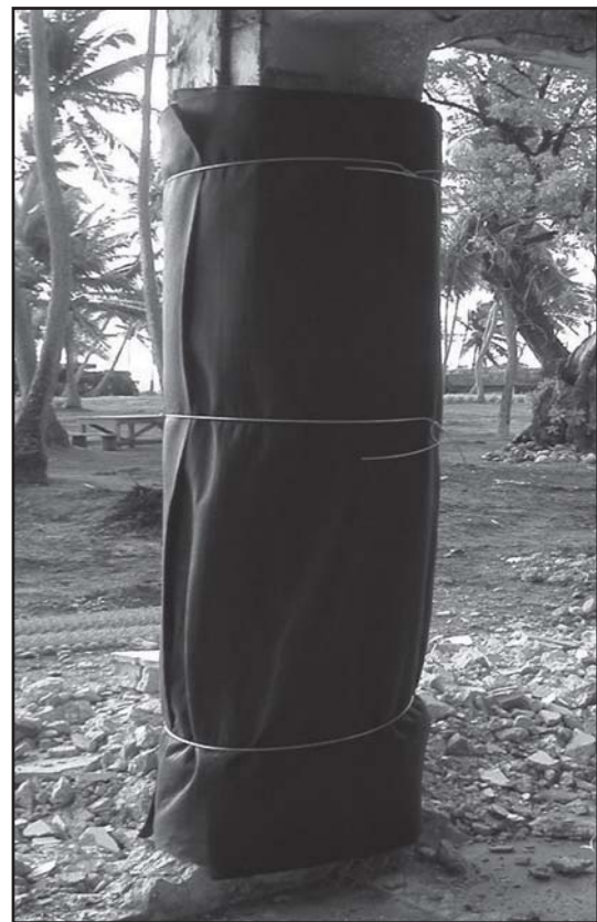
Each column was wrapped with two layers of chain-link fence and nonwoven geotextile fabric to contain fragmentation.
