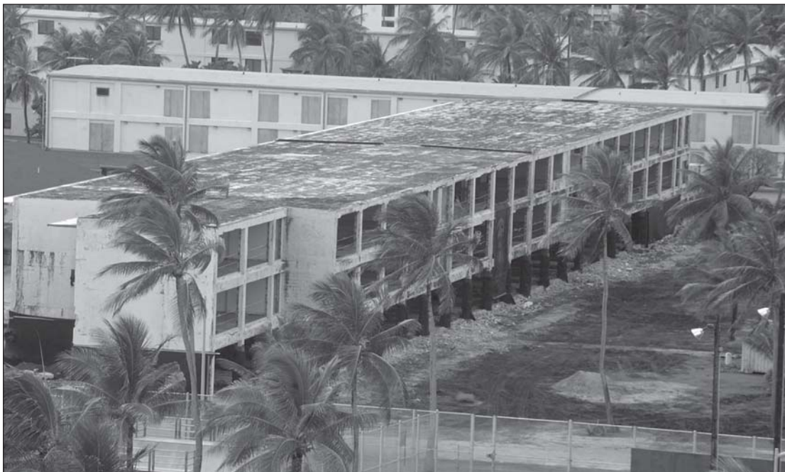
Glass and other interior components were removed from Building 708 in preparation for the implosion.
