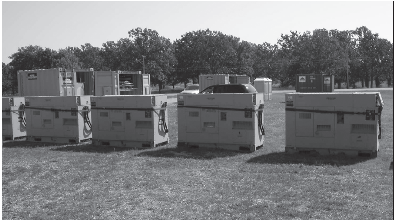
The ELSS generators can power the entire base camp.
