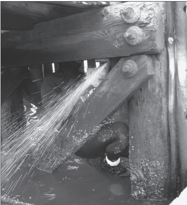
A hydraulic grinder is used to cut off rusted bolts before removing a support board.
