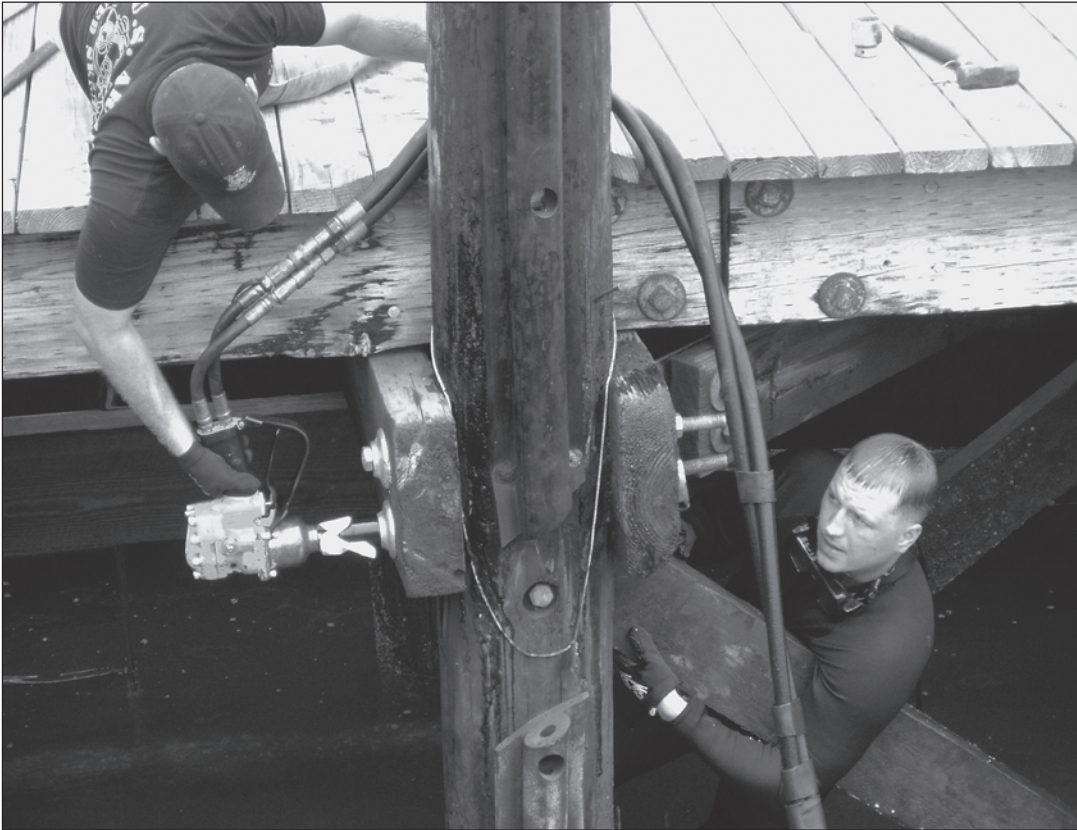
One diver uses a hydraulic impact wrench to tighten a board in place while another holds the hardware in place from the other side.
