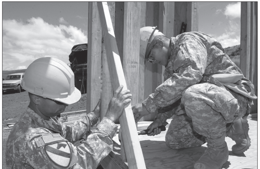
Soldiers from Alpha Company, 411th Engineer Battalion, construct a range house/observation tower during their annual training.
