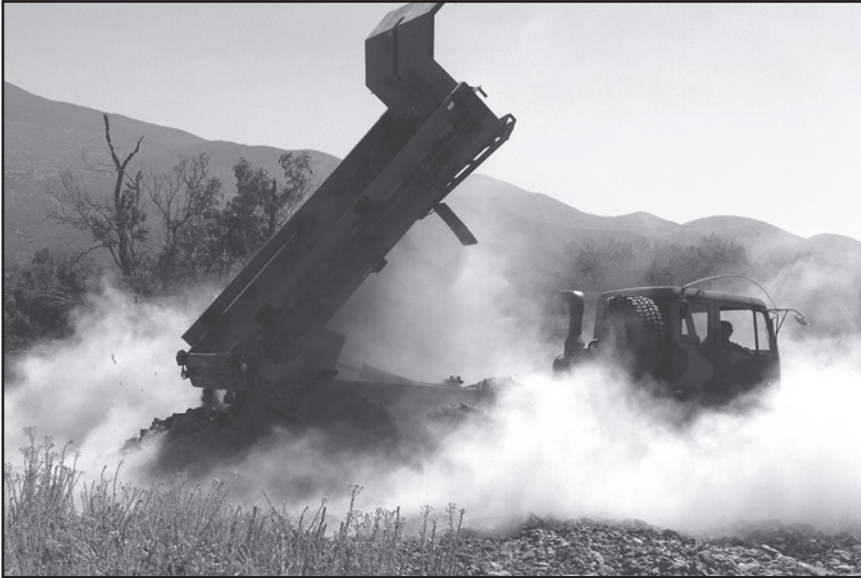
A load of freshly-crushed rock is dumped on a new road being built at Pohakuloa Training Area.
