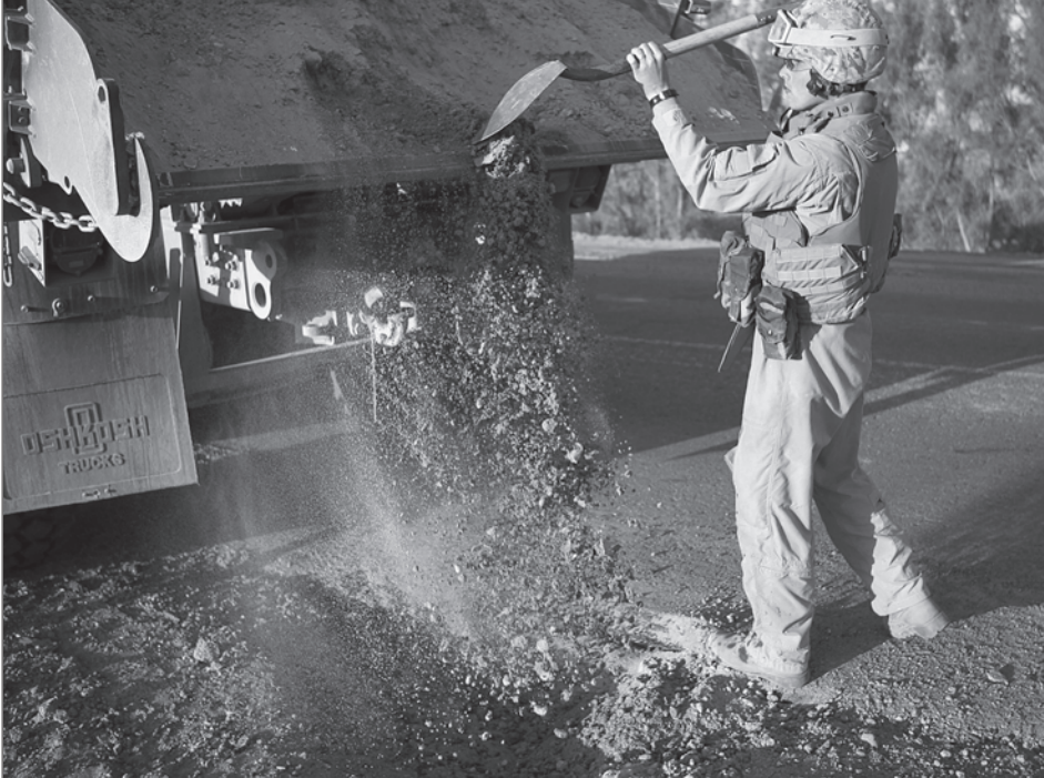
Left: A Marine shovels dirt from the back of a dump truck during a route repair mission.
