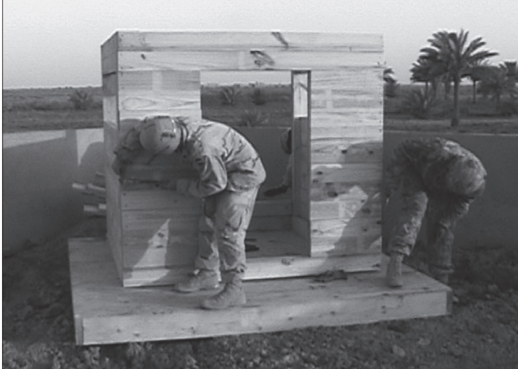
Soldiers from Alpha Company, 46th Engineer Battalion, construct the framework for guard positions.
