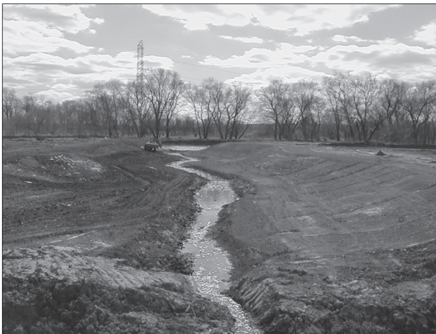
The banks of the "Finderne Brook"—that flows into the Raritan River—have been contoured to prepare for planting.
