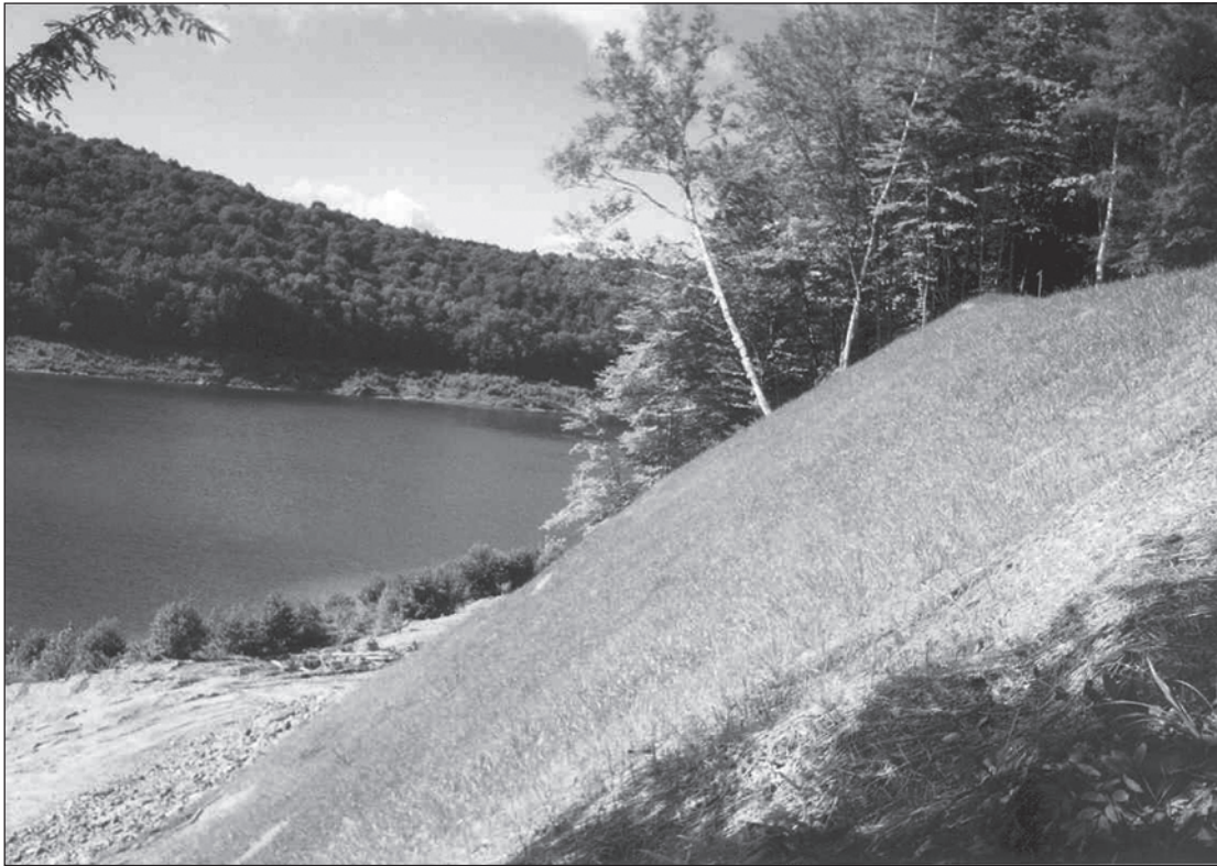
Riprap was placed at the bottom of the slope for stabilization, and the regraded slope was covered with grass seeding prior to fall plantings.
