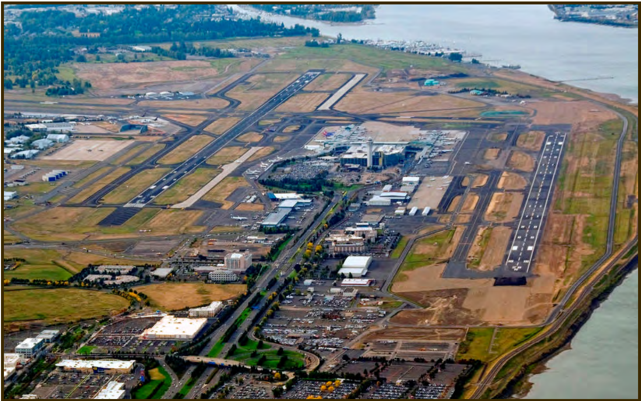
Portland International Airport Showing Runway 10L-28R extension under construction Photo courtesy of Port of Portland
