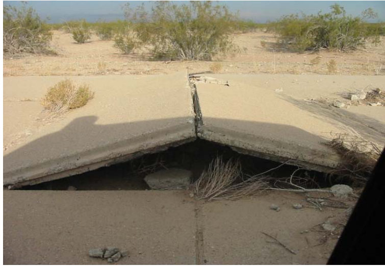
In addition to being a serious safety issue, the pavement at this airport inspected by the FAA needs obvious repair. Letting airport pavement deteriorate to this level is inconsistent with the sponsor’s grant assurances. (Photo: FAA)
