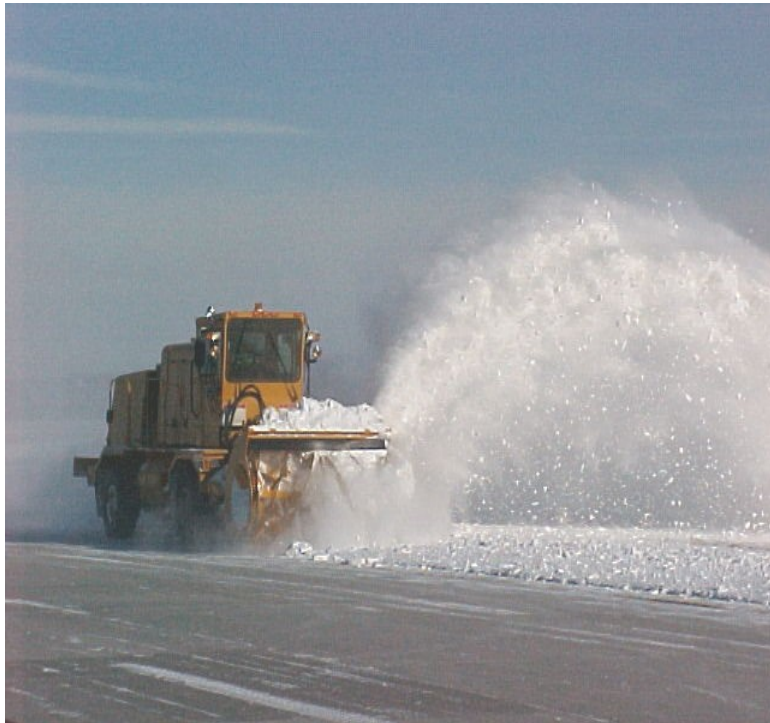
A sponsor's obligation to maintain the airport does not impose any specific responsibility to remove snow or slush or to sand icy pavements. To the extent possible, snow removal should be accomplished in those areas where public access is more likely. The sponsor, however, is responsible for providing a safe, usable facility. Where climatic conditions render the airport unsafe, the airport sponsor must promptly issue a Notice to Airmen (NOTAM). (Photo: FAA)
