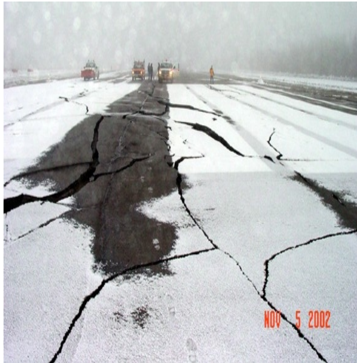
The obligation to maintain the airport does not extend to major rehabilitation of a facility that has become unusable due to normal and unpreventable deterioration or through acts of God, including earthquakes, as seen here in Alaska in 2002. Northway (ORT) runway was destroyed by a 7.9 magnitude earthquake. (Photo: FAA)
