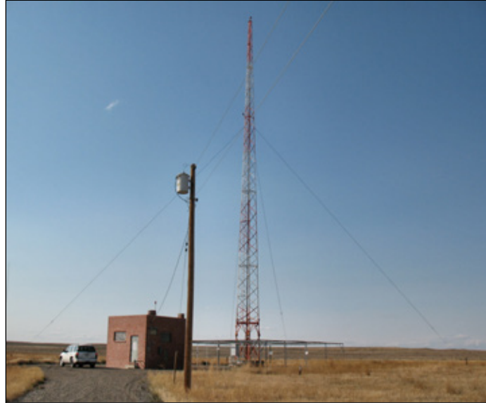
Figure 6-31. Non-Directional Beacon (NDB) facility
