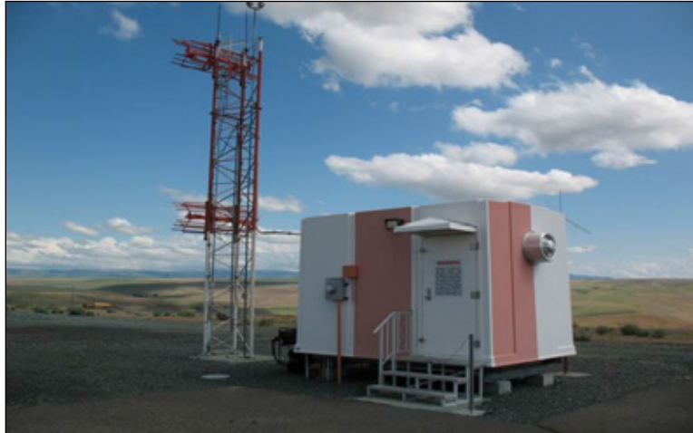
Figure 6-24. GS antenna and equipment shelter
