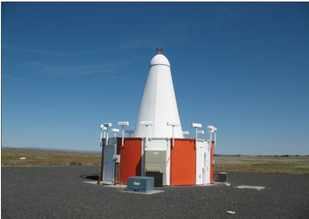
Figure 6-28. Terminal VOR (TVOR) facility
