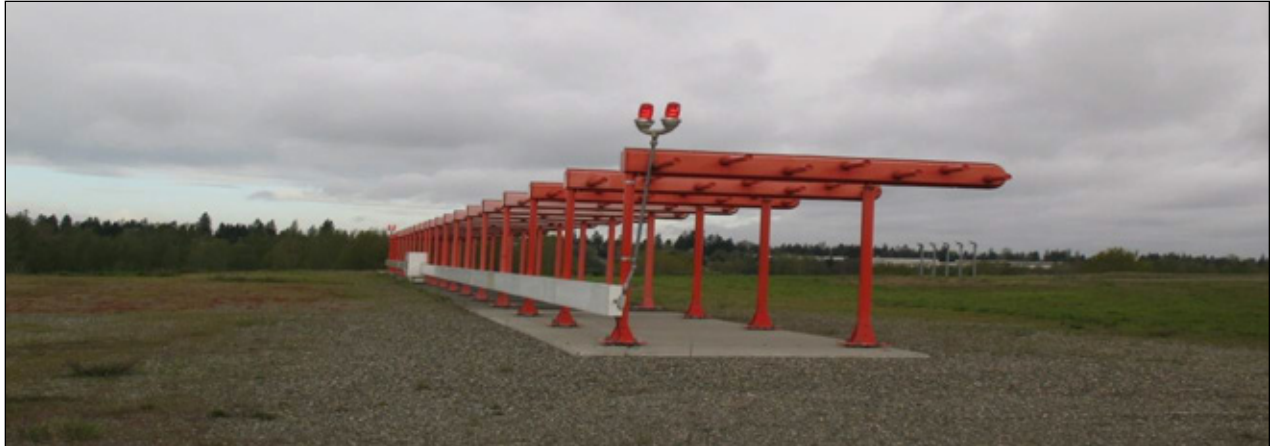
Figure 6-22. LOC 14-antenna array
