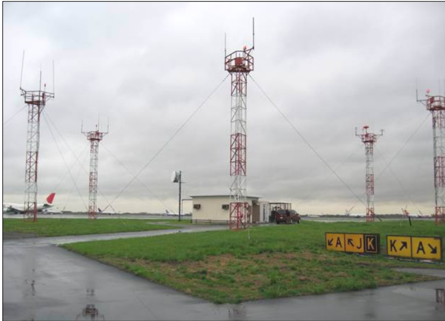
Figure 6-4. Remote Transmitter/Receiver (RTR) communication facility
