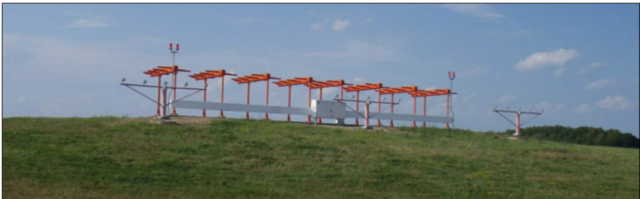
Figure 6-21. LOC 8-antenna array
