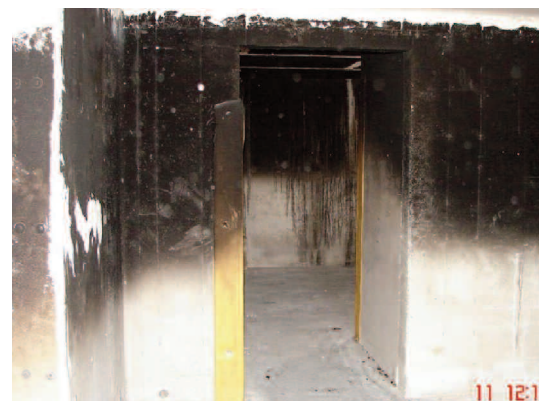
Figure C-7: Interior View of Burn Prop
