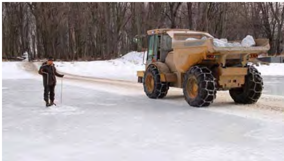
As refuge biologist Judy Sefchick-Edwards closely monitors conditions, a dump truck carries tons of rip-rap on an ice bridge that equipment operator Joe Bertrand built at Missisquoi National Wildlife Refuge in Vermont to transport rock across the Missisquoi River for a project to conserve a Native American cultural site. (Ken Sturm/USFWS)
