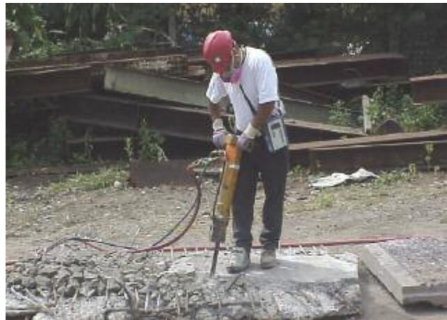
Employee chipping concrete with a jackhammer while using a wet method. (Photo courtesy of NIOSH.)
