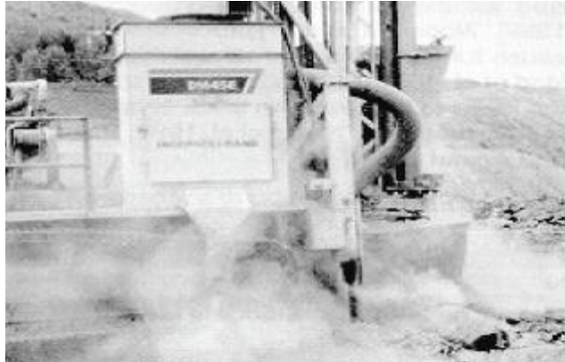
Earth drilling rigs operated without dust controls are capable of producing very high respirable silica levels (Photo courtesy of NIOSH, 1992.)
