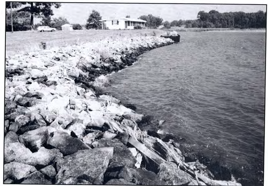
Figure 38. Riprap revetment is preferred over bulkheads for shore stabilization in the Bay (USFWS photo).
