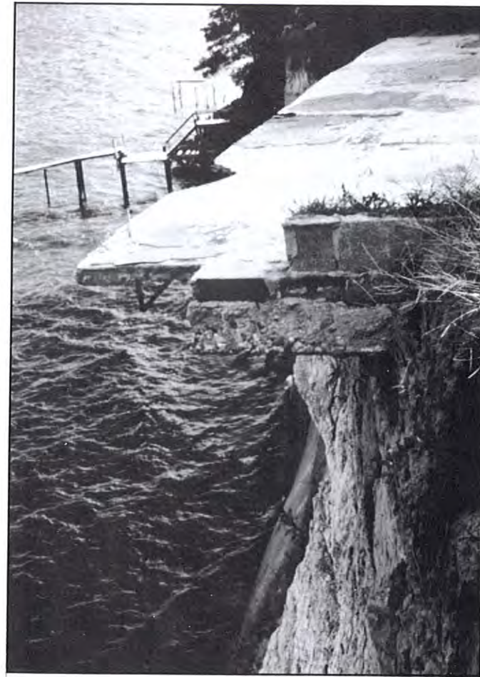
Figure 25. Erosion of the Western Shore cliffs has resulted in loss of houses (Randle Cliffs area) (photo by Stephen Leatherman).
