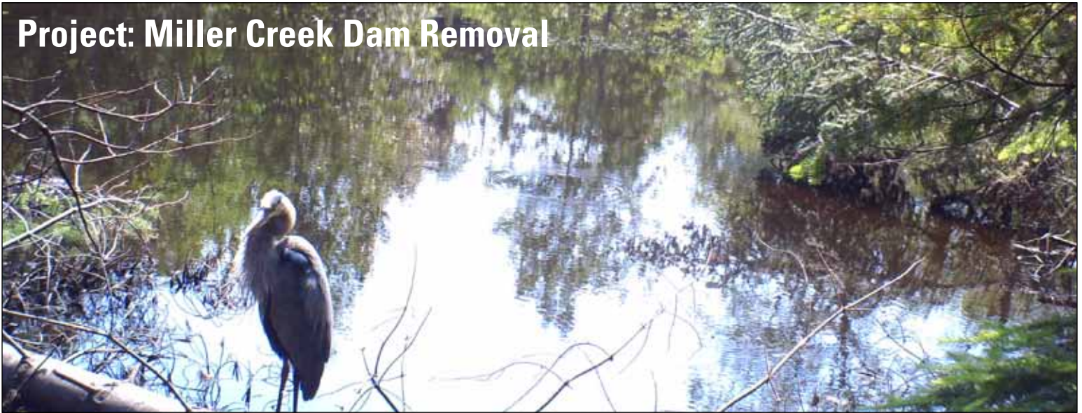
View of Miller Dam impoundment approximately one month after the concrete base was removed. The stream channel began to form immediately following removal and the area is beginning to vegetate. USFWS
