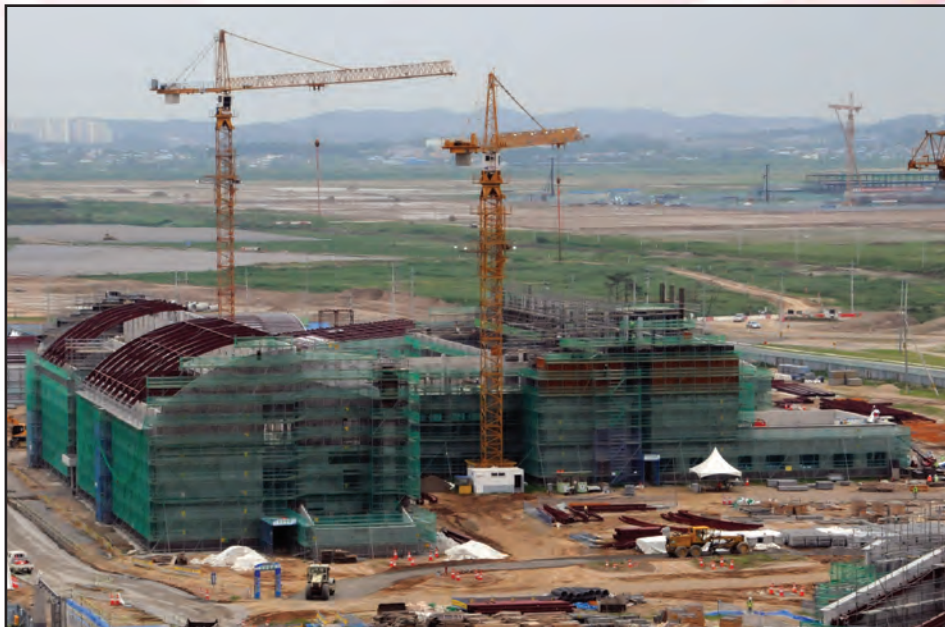
(Below) The high school project currently underway at U.S. Army Garrison Humphreys is a quality of life project by the Far East District and managed by the Korea Program Relocation Office. (Photo by Patrick Bray)
