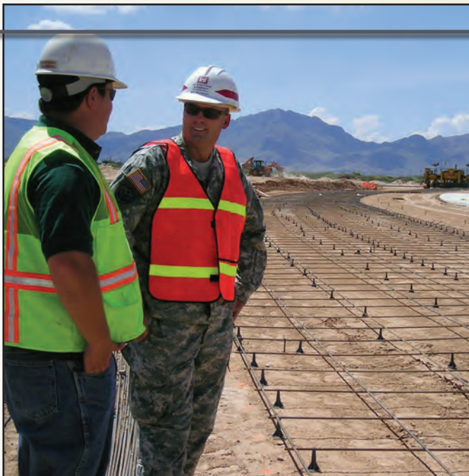
Sgt. Major David Breitbach (right), FED Sergeant Major, looks over a road extension project at Ft. Bliss, Texas prior to his assignment at FED. Breitbach enjoys being an engineer and the many exciting projects that come along with the job. (Photo provided by Sgt. Major Breitbach)
