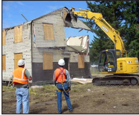
Workers remove the building in partitions to maximize recovery during the deconstruction project at Fort Lewis.
